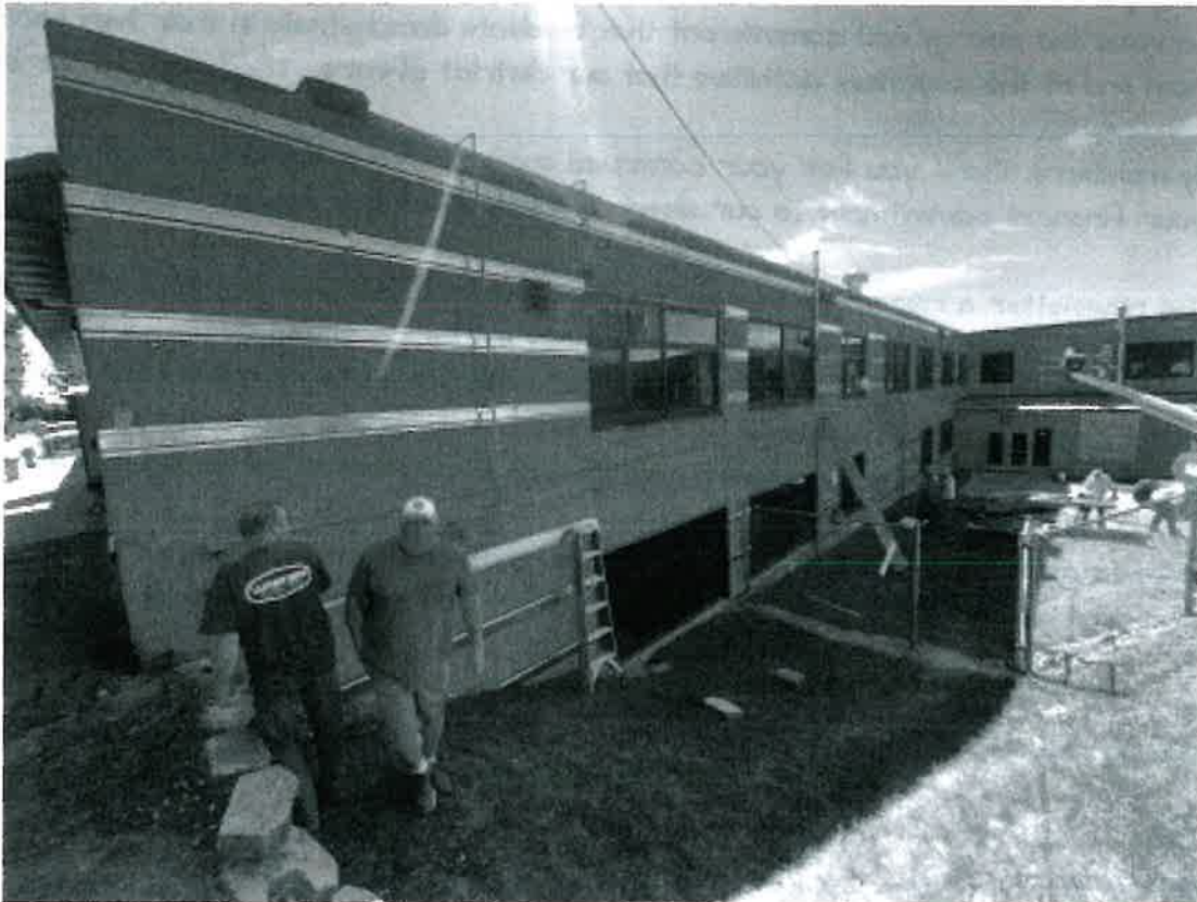
Electrical & Gas Contractors are onsite to remove conduit away from the side of buildings.
