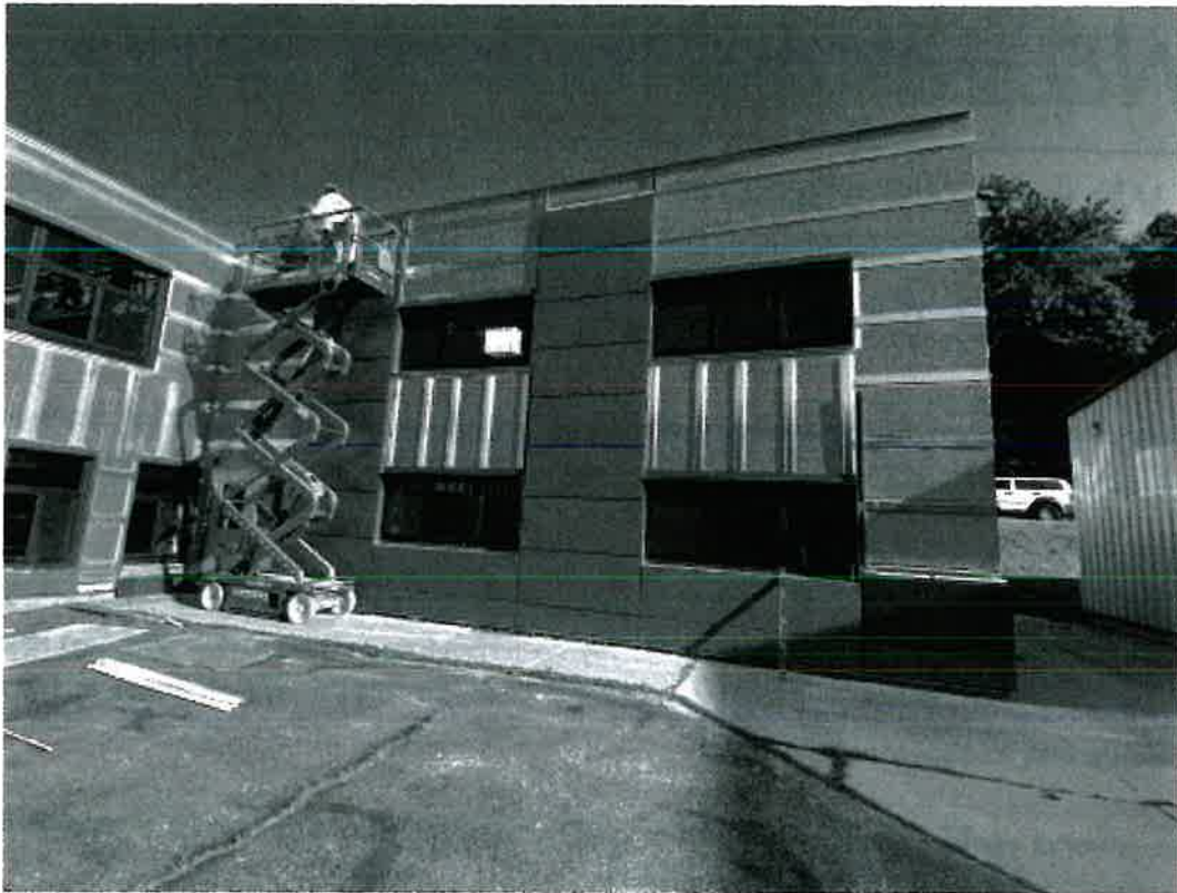
Courtyard Progress – Liquid Vapor Barrier is installed; Hat Channels and Window Trims are set in place. Various panels are dry fit near window openings to ensure proper fit.
